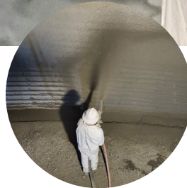
For this repair job, the existing dome was used as the concrete form for a new concrete dome.
