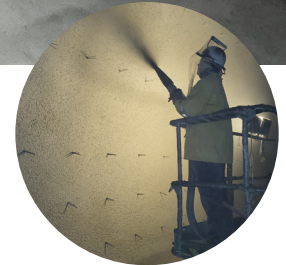
New concrete was applied inside the existing dome using the shotcrete method.
