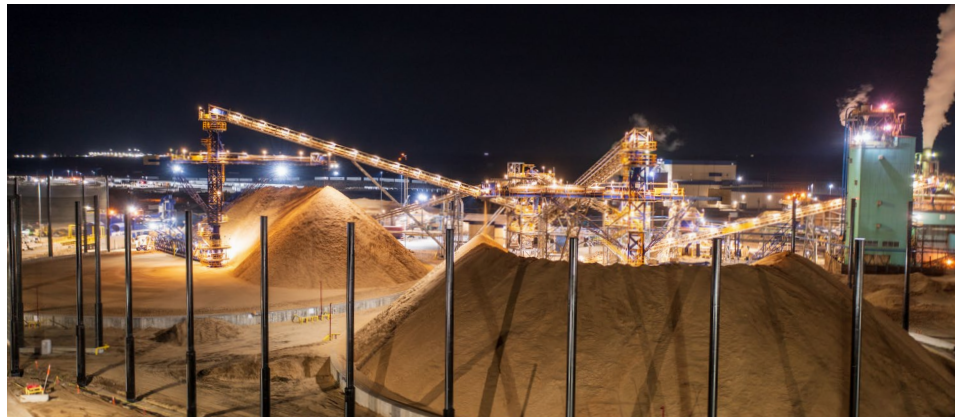
Installation of foundation systems, including ring beams, fell within Dome Technology's scope of work.
