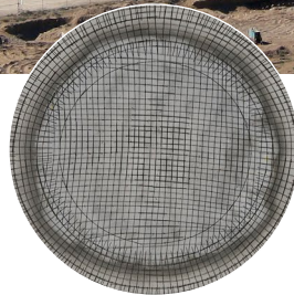
This image shows the grid of rebar placed at the roof apex atop insulation.
