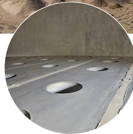
Multiple hoppers in the dome floor feed sugar onto at-grade conveyor belts.
