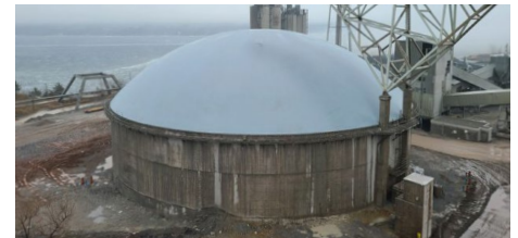
The new dome with its PVC covering will add decades of life to the existing concrete silo.
