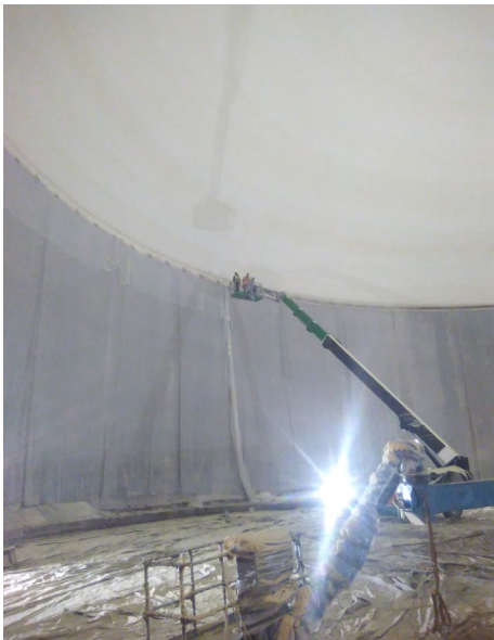
After the airform is inflated, crews apply concrete to the inside of the PVC form using the shotcrete method. When complete, the monolithic dome is leak proof.
