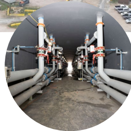
A single tunnel under the DomeSilo houses the aeration valves and pipes.
