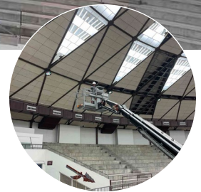
The team designed all steel components around preserving the existing star motif in the dome roof.
