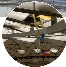
Fabricated in the Dome Technology shop, new steel beams were installed below the existing wood beams.
