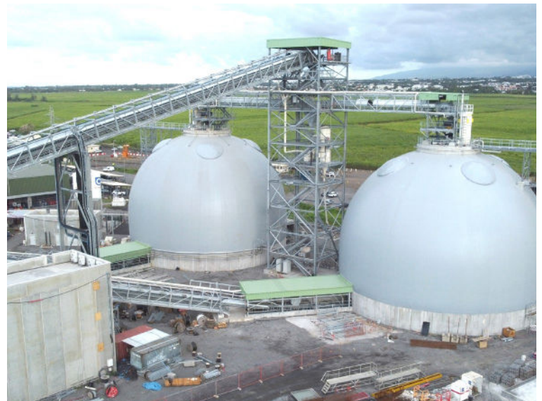
Albioma's two new domes feature round explosion venting, like their dome in Martinique.
