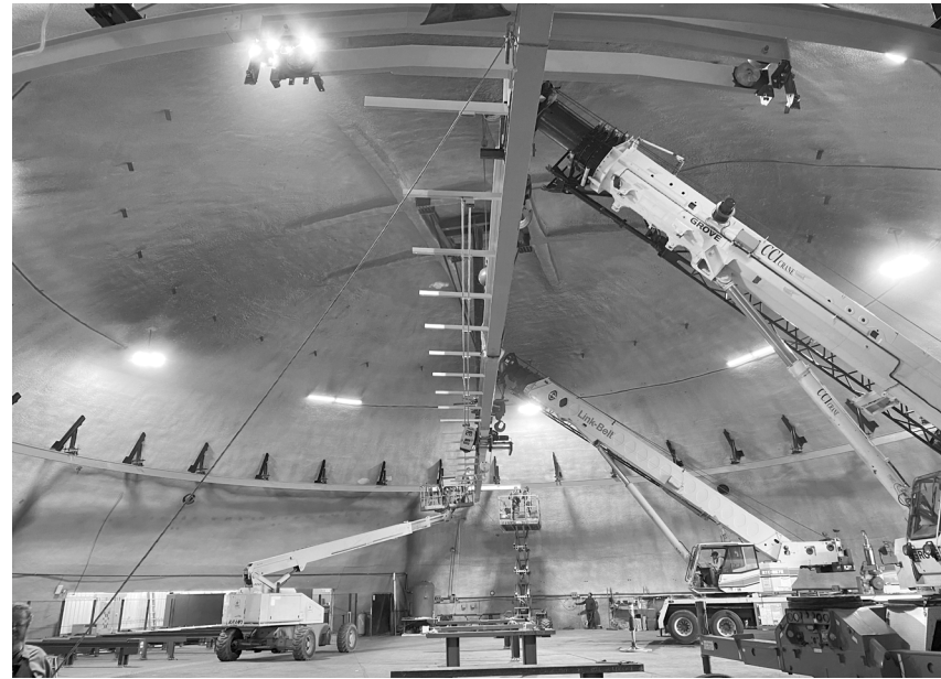
A crane installed in 2020 increases the ability to move steel during work.
